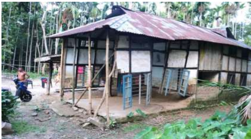
Pic: Houses washed out by the sudden rising water of Kopili River at Gosaigaon Village, Assam
