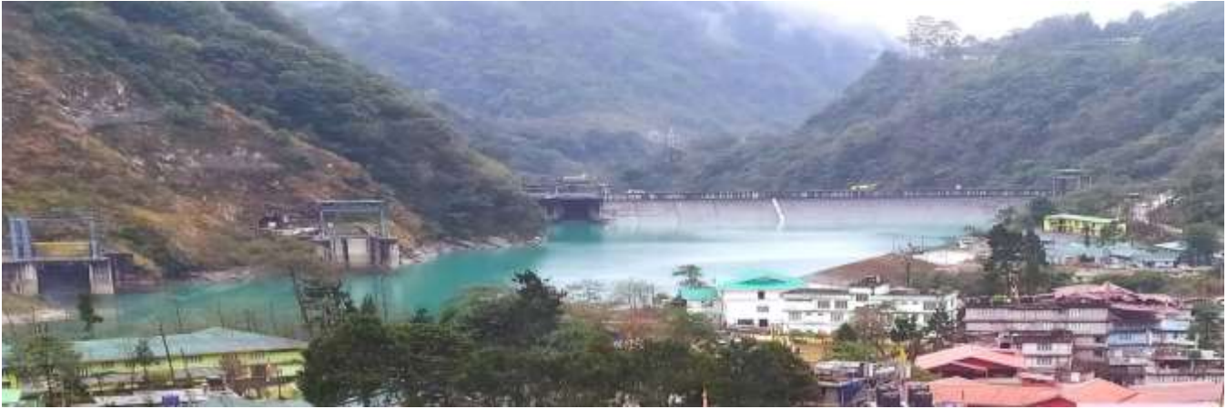
Pic: The dam site of 1200 MW Teesta III Hydroelectric Project at Chungthang Village, North Sikkim
